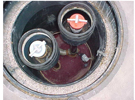
Sump that contains the spill buckets
