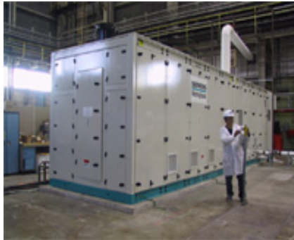
250 kW CHP System Canada
