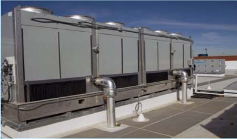
Fluid Cooler on Roof
