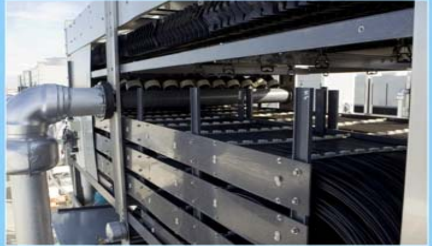
Piping Racks provide Extended Cooling Surface
